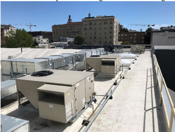
Third Floor Roof mounted equipment
