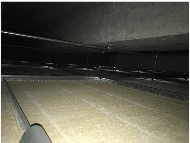
Third Floor Suspended Ceilings with Wire Bracing
