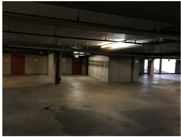
Building Basement & MEP Bracing
